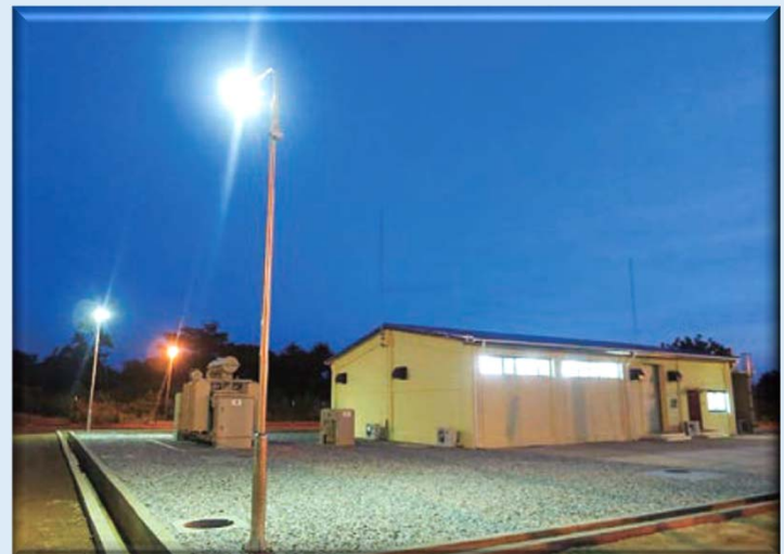
Kotokrom Primary Substation
