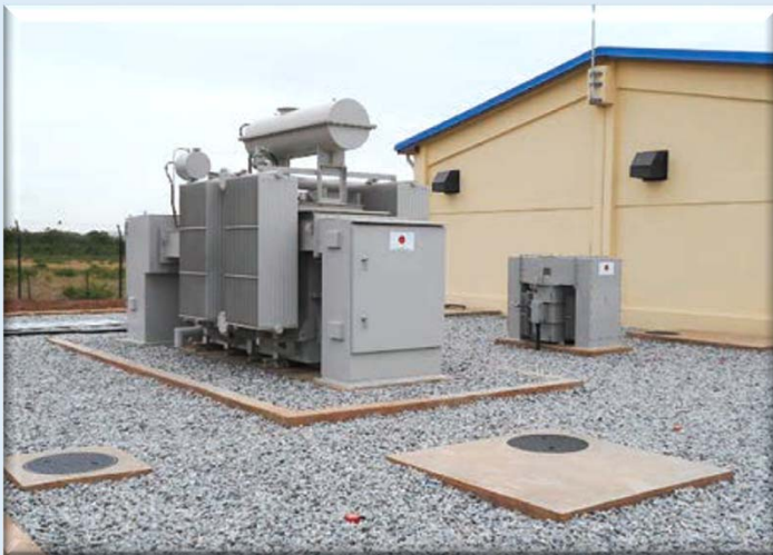
UDS Primary Substation
