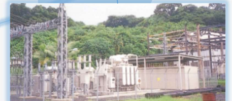
Palau Project (34.5/13.8kV AIS, etc.)
