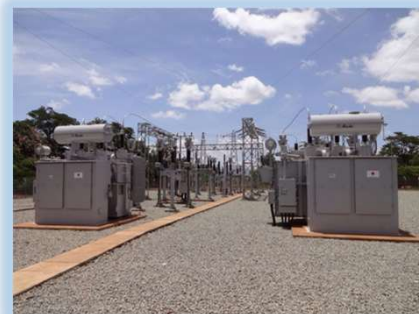
Tanzania Project, 2013 (66/33kV 10MVA x 2 AIS, etc.)
