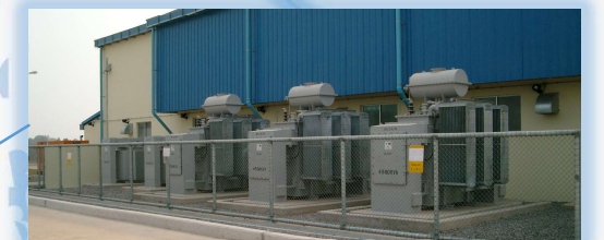
Cambodia Project, 2004 (DG P/S electrical system)
