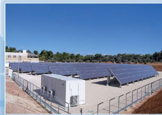
Jordan Project, 2011 (280kW solar P/S)
