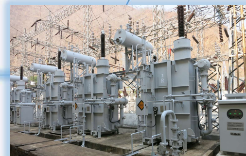
Myanmar Project, 2016 (11/132kV 10MVA x 18, etc.)
