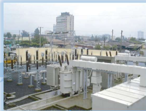
Ethiopia Project, 1997 (132/15kV 31.5MVAx2 AIS)
