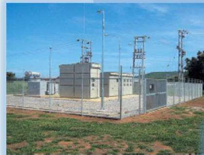
Nigeria Project, 2001-2010 (Rural Electrification)
