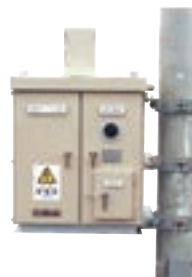
Signal line transformer panel (mounted on a pole)
