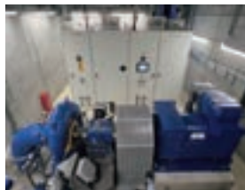
Hydropower turbine, generator and control panels
