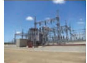
Completed Namialo Substation
