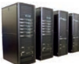
Master station servers (at one location)
