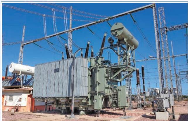
275/66/11kV 250MVA Auto-transformer
