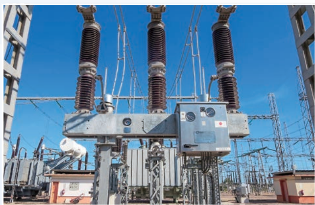
66kV Circuit Breaker
