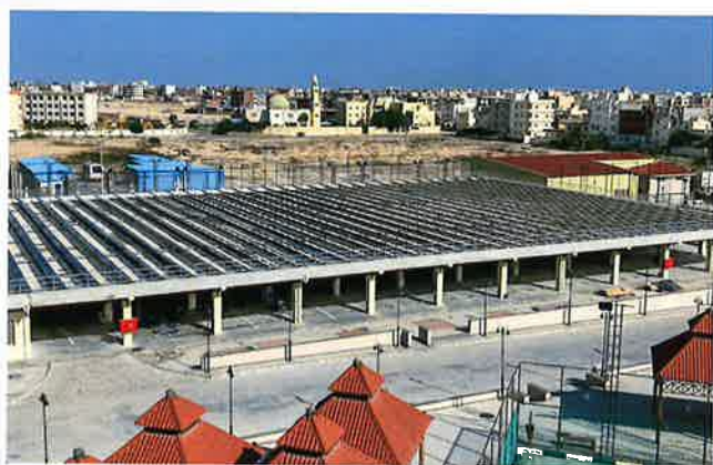
PV modules at Parking
