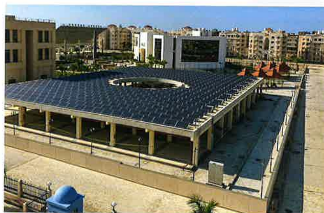
PV modules at Plaza
