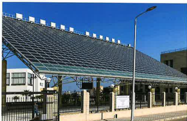
PV modules at Atrium
