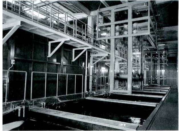
図6/前処理・電着装置 Fig. 6/Pre-treatment and electrodeposition equipment
