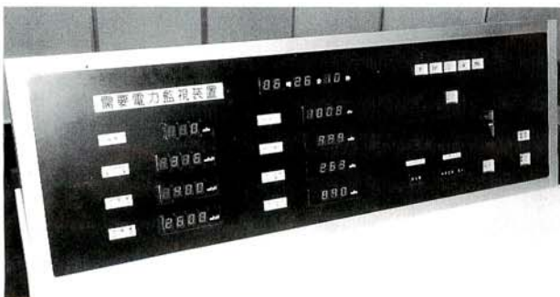
図4/監視パネルの外観 Fig. 4/Exterior of supervising panel
