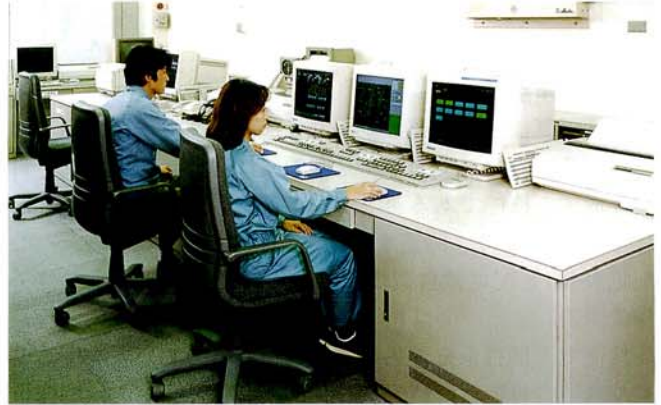
図10/親局操作卓 Fig.10/Operation console
