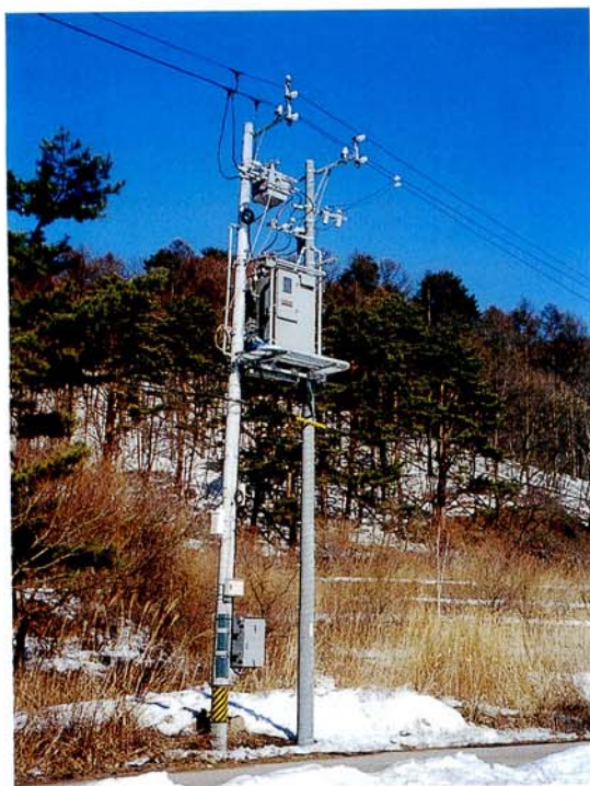
図10 SVCの装柱風景 Fig. 10. View of SVC mounted on pole
